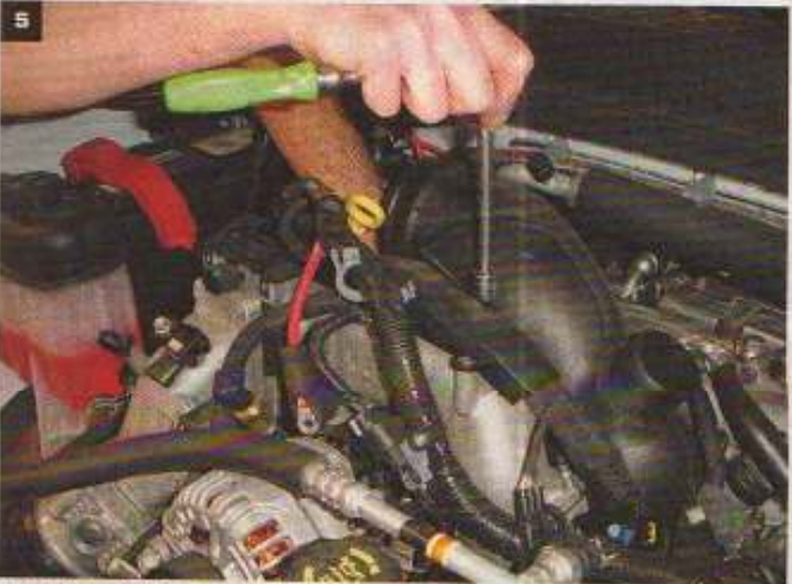
Removing the factory air intake provided access to the bolts that secure the aluminum intake.
